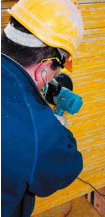
Wood grinding approx. 90 dB
