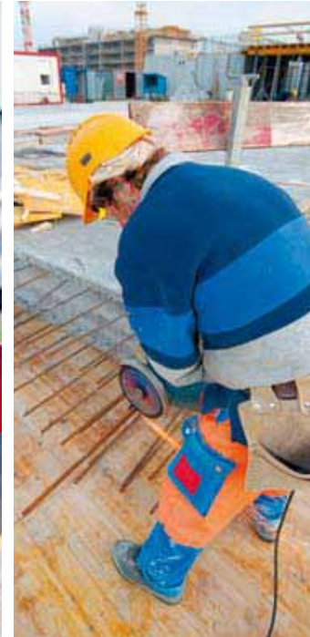
Separation grinding machine approx. 110 dB
